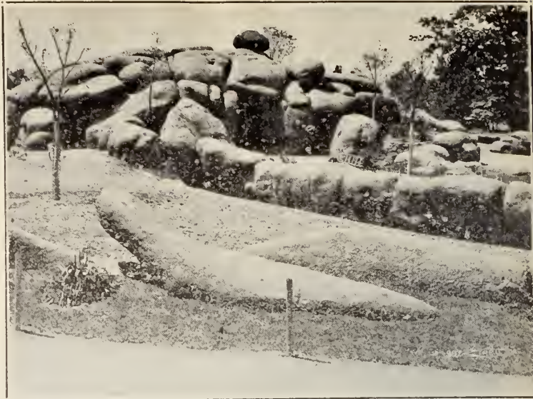
5. Showing finish coat of ground red granite and cement which was applied with cement guns. Completed, these groups look exactly like boulder groups in their natural state. This photo shows only part of one side of one building. Note dividing walls also built of boulders.
